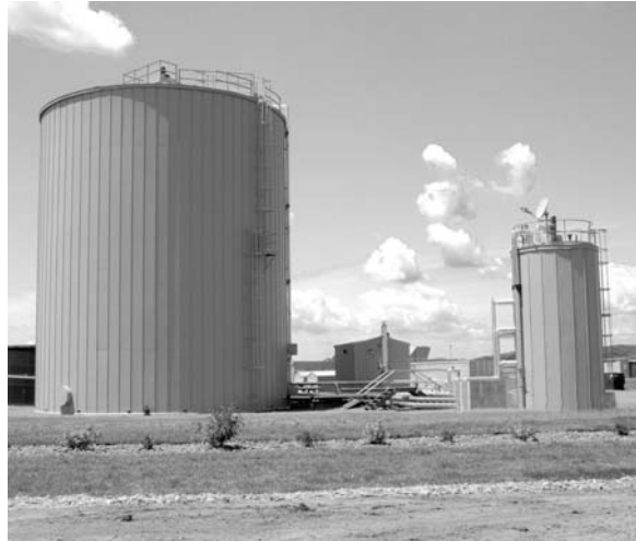
The EPG digester system installed at Five Star Farm
